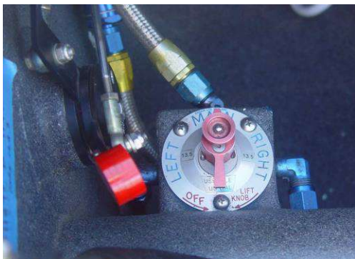
Fuel switch in ON position.
